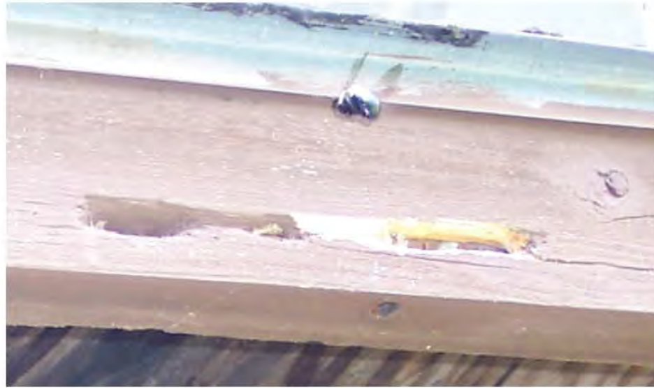
Figure 1-6. Carpenter bee and its damage.
